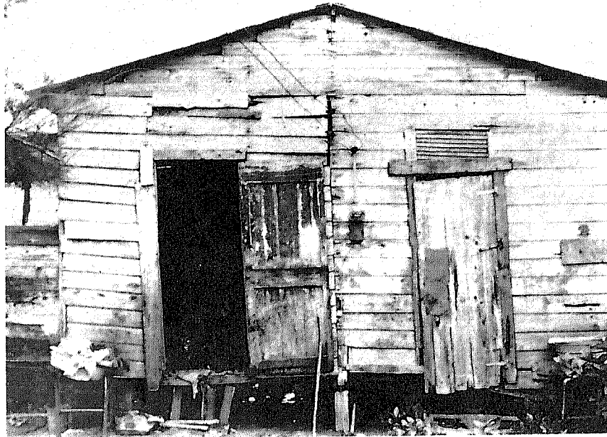
Figure 3. A dilapidated house no longer provides safe and adequate shelter. It endangers the health or well being of the occupants.
