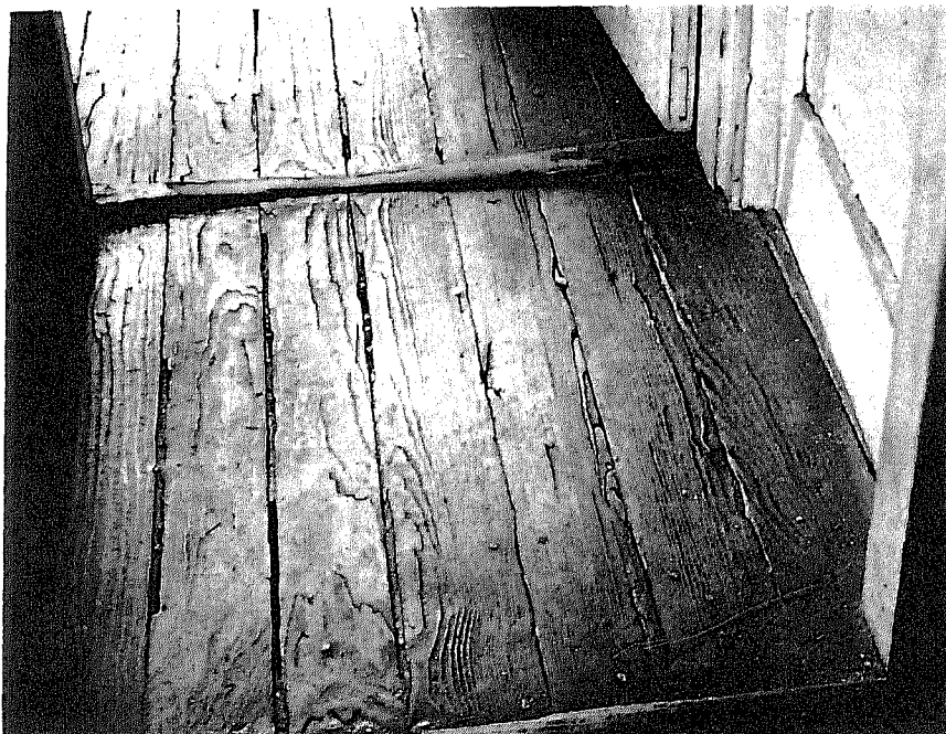
Figure 9. Deeply worn floors and doorsills are intermediate defects. They are signs of deterioration.
