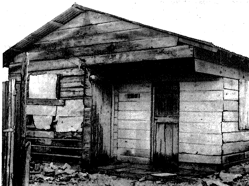
Figure 20. A house without a foundation is not adequately built. This house rests directly on the ground and the wooden siding is beginning to rot. Mark it inadequate original construction.
