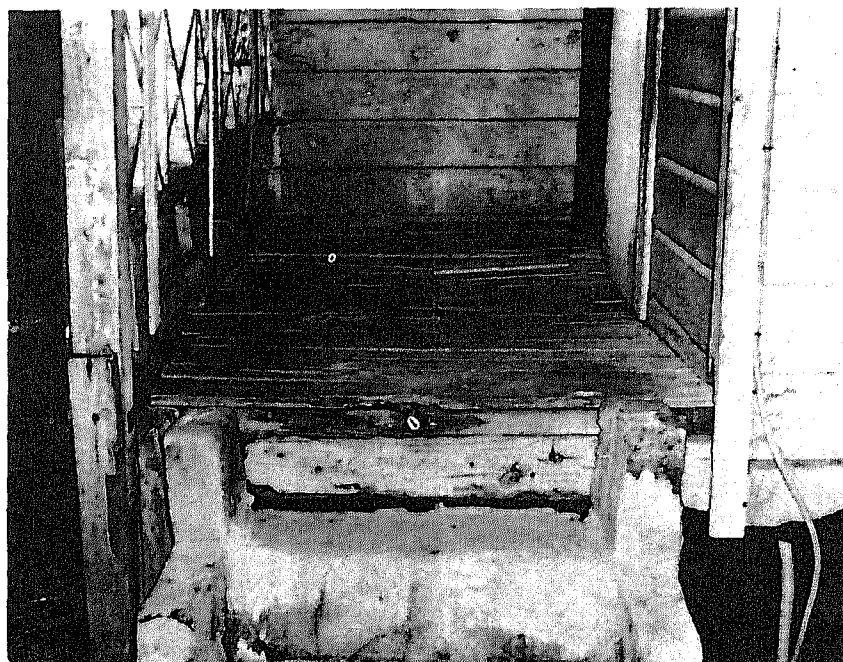
Figure 10. Here the porch and steps are rotted and unsafe. Whenever you see intermediate defects, however, watch for other defects that may indicate the house no longer provides safe and adequate shelter and is therefore dilapidated.
