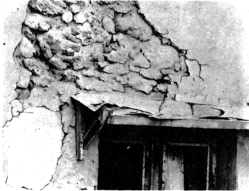
Figure 11. A house is dilapidated if it has one or more critical defects. This large area of broken and missing material is critical because it is a sign of structural damage you cannot see.
