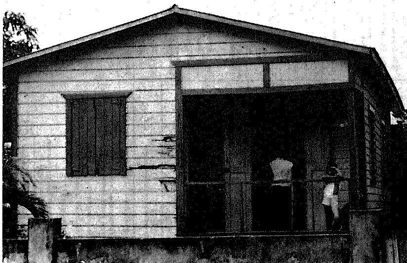
Figure 2. A deteriorating house needs more repair than is provided by regular upkeep. This small area of rotted material is a sign of neglect or damage.
